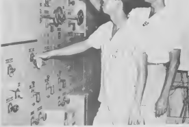
SWITCHBOARD POINTERS are give to C. N. Chang, foreground, U.T.S. student on a recent training assignment in Process-Utilities, by Z. E. Preston, Foreman at No. 1 Powerhouse. INSTRUMENT FIXER ANSTE and switchboard man, José C. N. Chang, assistant, estudiante di U.T.S. cu ta cumpliendo un periodo di entrenamiento na Process-Utilities, door di Z. E. Preston, operator na No. 1 Powerhouse.
